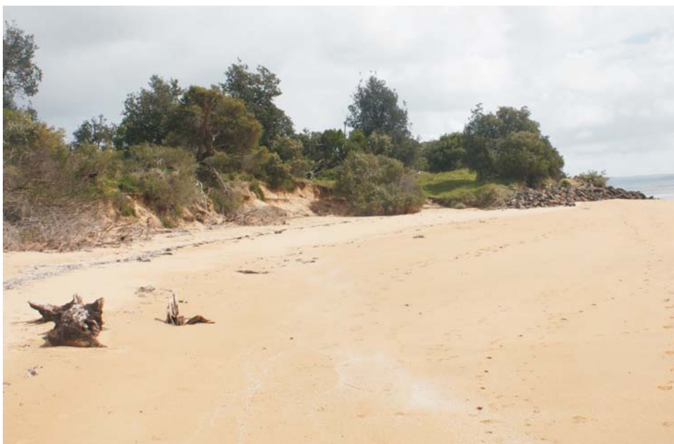
Above: The rock wall (right) must be extended if this foreshore is to be saved.
