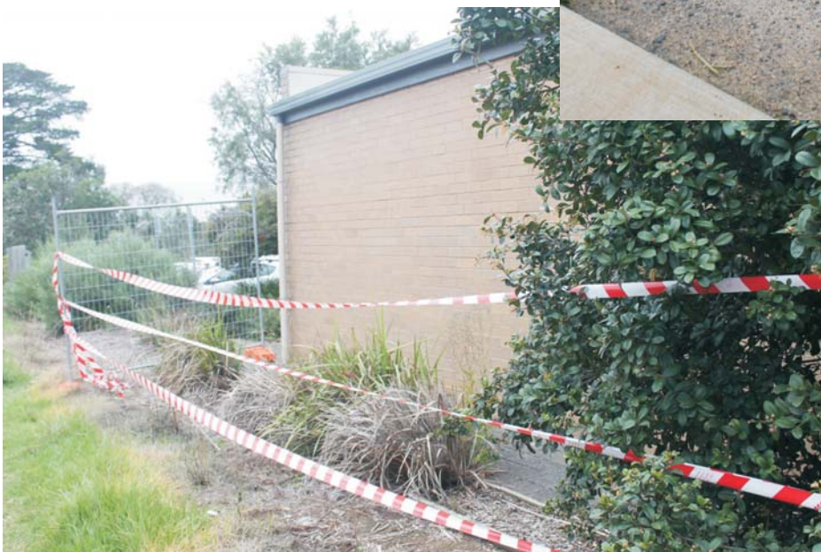
Left: Condemned brick wall, Cowes Heritage Centre. Over 12 months and no action taken.
